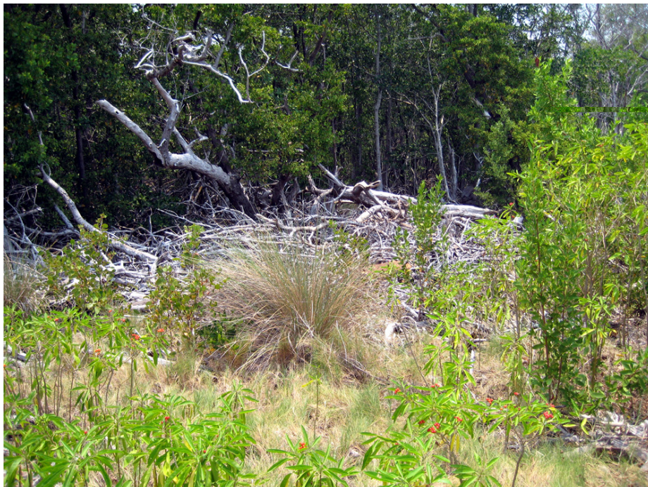
Figure 6. An airstrip recently constructed on southern Blackbird Cay (top). Debris (primarily dead mangrove) from airstrip construction piled atop a former American crocodile ( Crocodylus acutus ) nest site.
